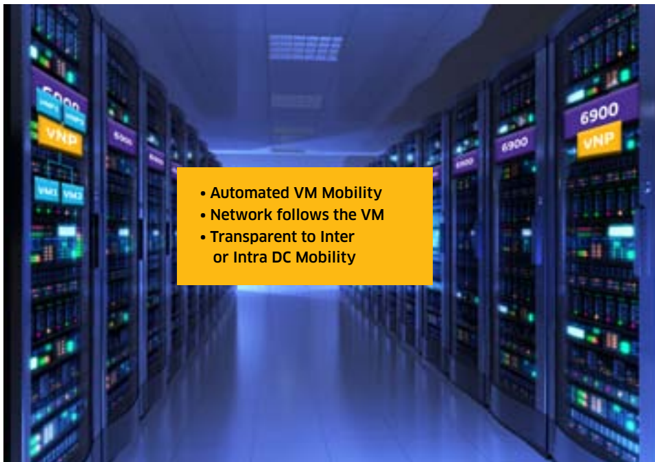
Figure 5. Virtual machines are identified by vNPs shared with all switches in a typical data center
