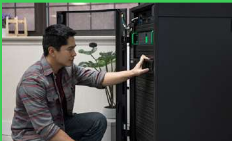
Micro Data Center
